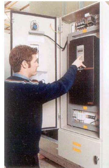
Factory-fitted variable speed drive, marshalling box and electrical cable trunking to customer requirements.
