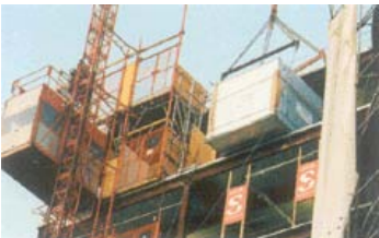
Lifting, positioning and installation of AHU's is all part of IAC's service.
