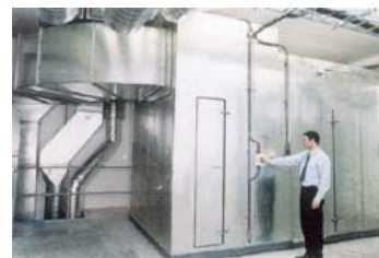
Typical, compact on-floor AHU
