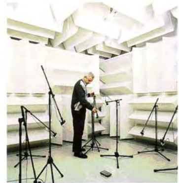
Metadyne® semi-anechoic component test room for IBM (Germany).
