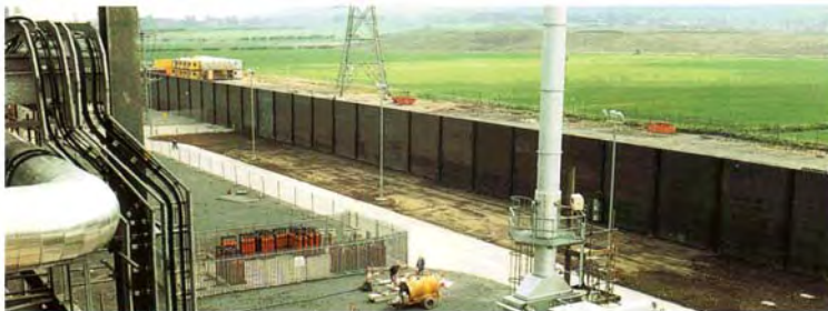
Noishield® acoustic barrier at Teesside Power Station.
