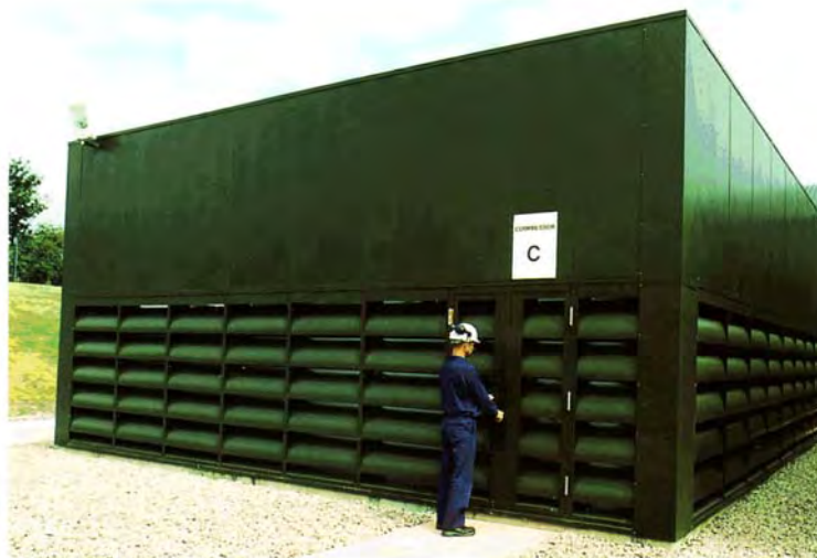
Noishield® acoustic louvres provide ventilation to the plant inside this IAC acoustic enclosure.
