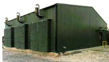
A 15m x 13m x 6m high Moduline® acoustic enclosure houses three 1MW gas engine generator sets.
