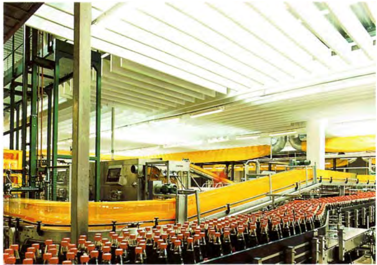
Ceiling-hung Varitone® sound absorptive panels reduce noise and reverberation in a Coca-Cola bottling plant.
